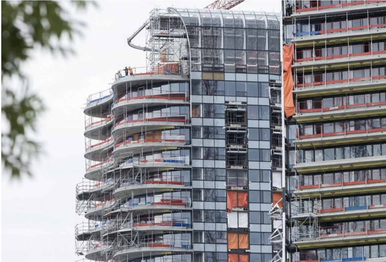
Condos under construction near Cambie and West 41st Ave. in Vancouver Photo by Arlen Redekop /PNG
