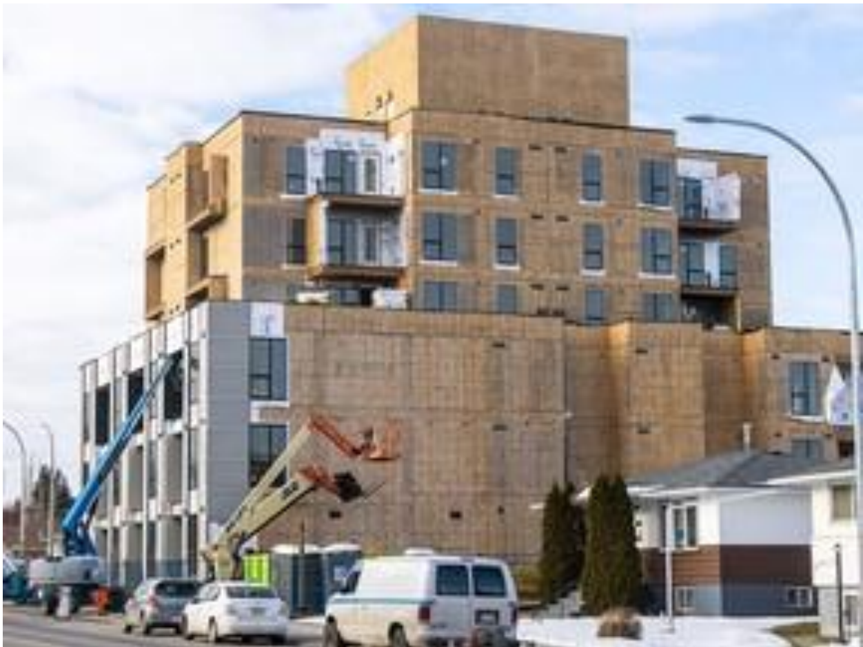
Multi-unit housing under construction on 24th Avenue N.W. in Calgary on Dec. 11, 2024. Brent Calver/Postmedia
